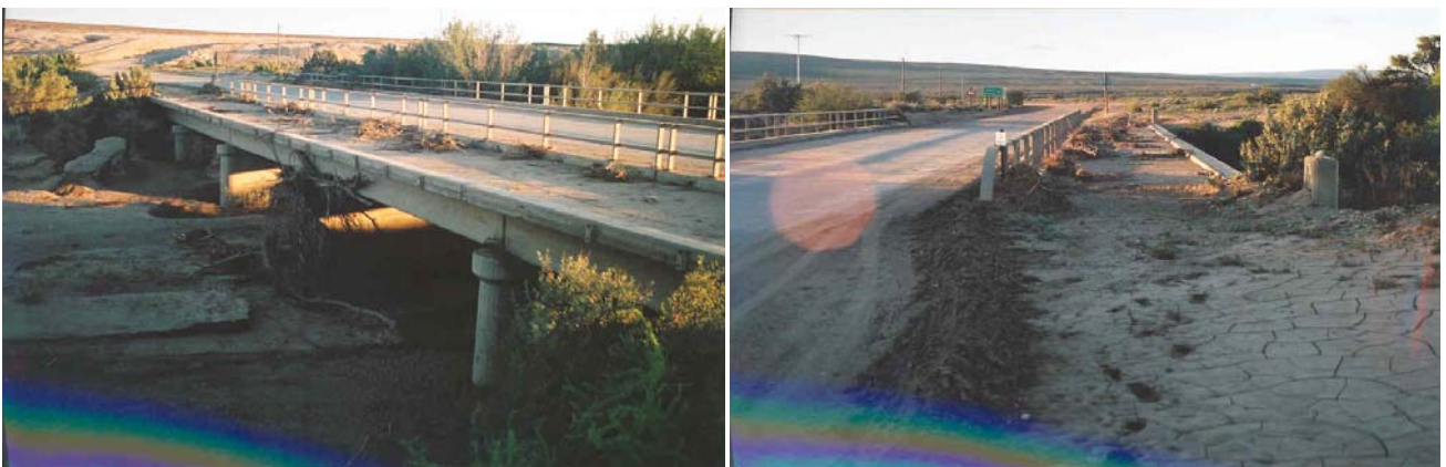
Figure 3.4 Debris on bridge over dry riverbed of the Hols River 24 April 2005.
